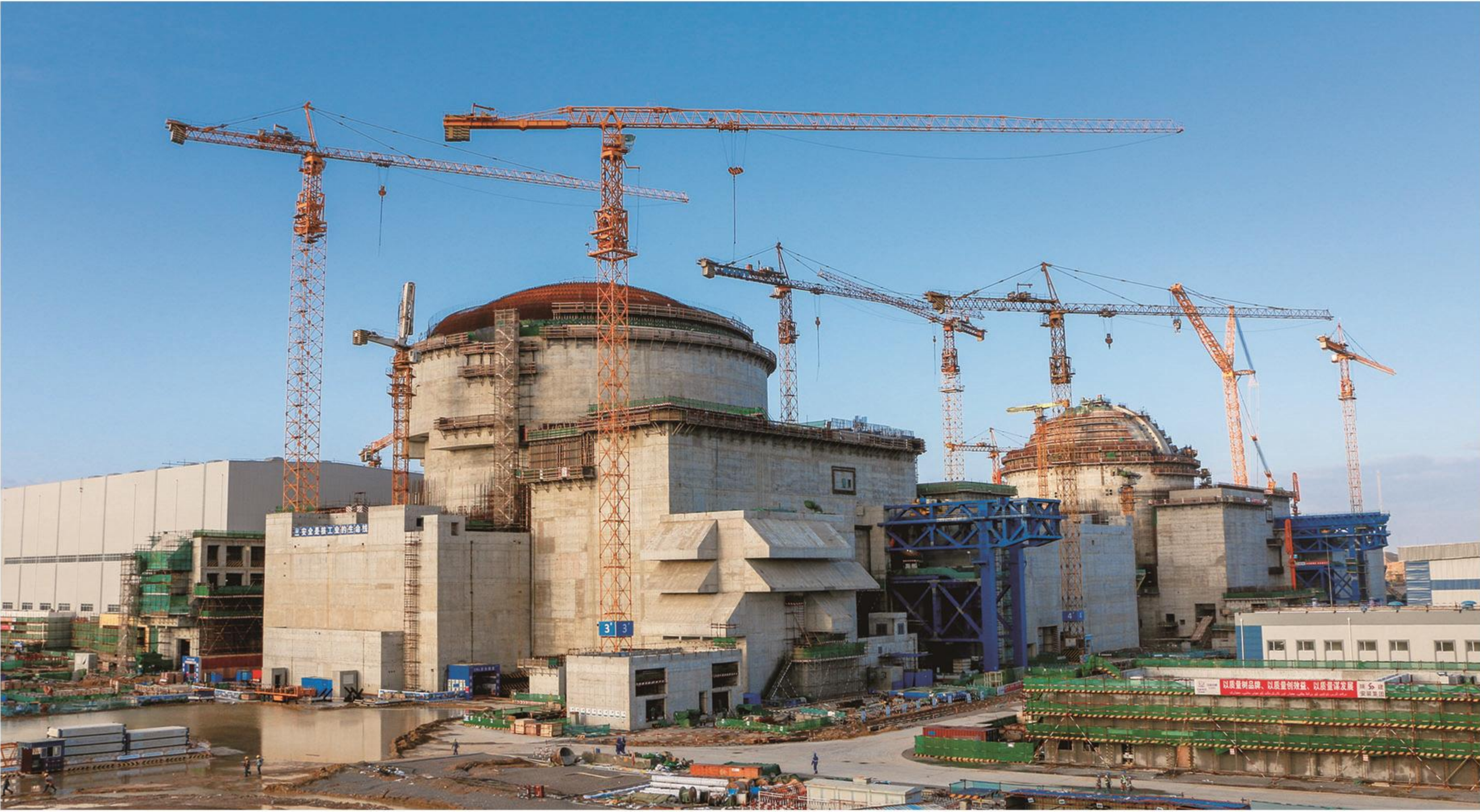
巴基斯坦卡拉奇核电站，我国出口海外的第一座“华龙一号” Pakistan Karachi Nuclear Power Plant, the first “Hualong One” exported by China to overseas
