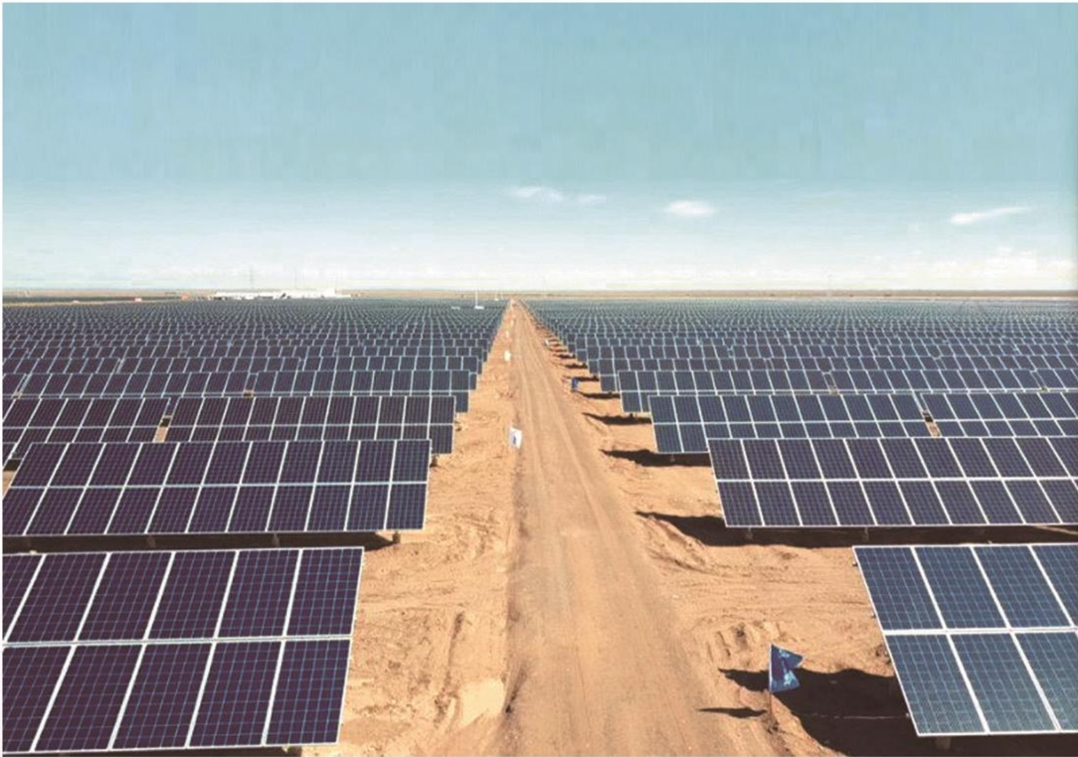
新疆木垒光伏园100MWp光伏发电项目 Xinjiang Mulei PV Power Garden 100MWp Photovoltaic power generation project
